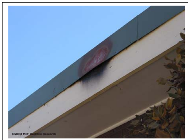
Figure 4 – Ember attack at an eve lining
