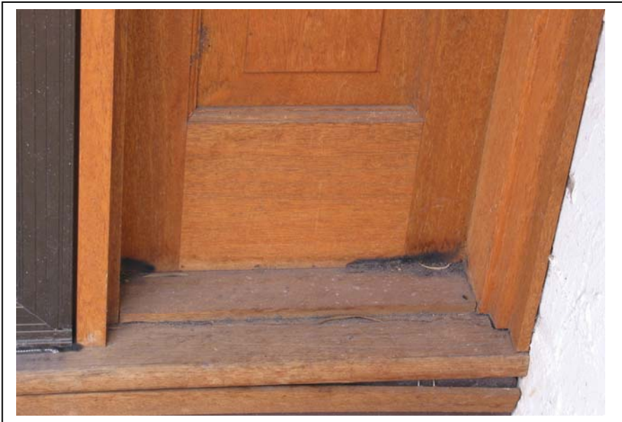
Figure 2 – Ember attack at a doorway
