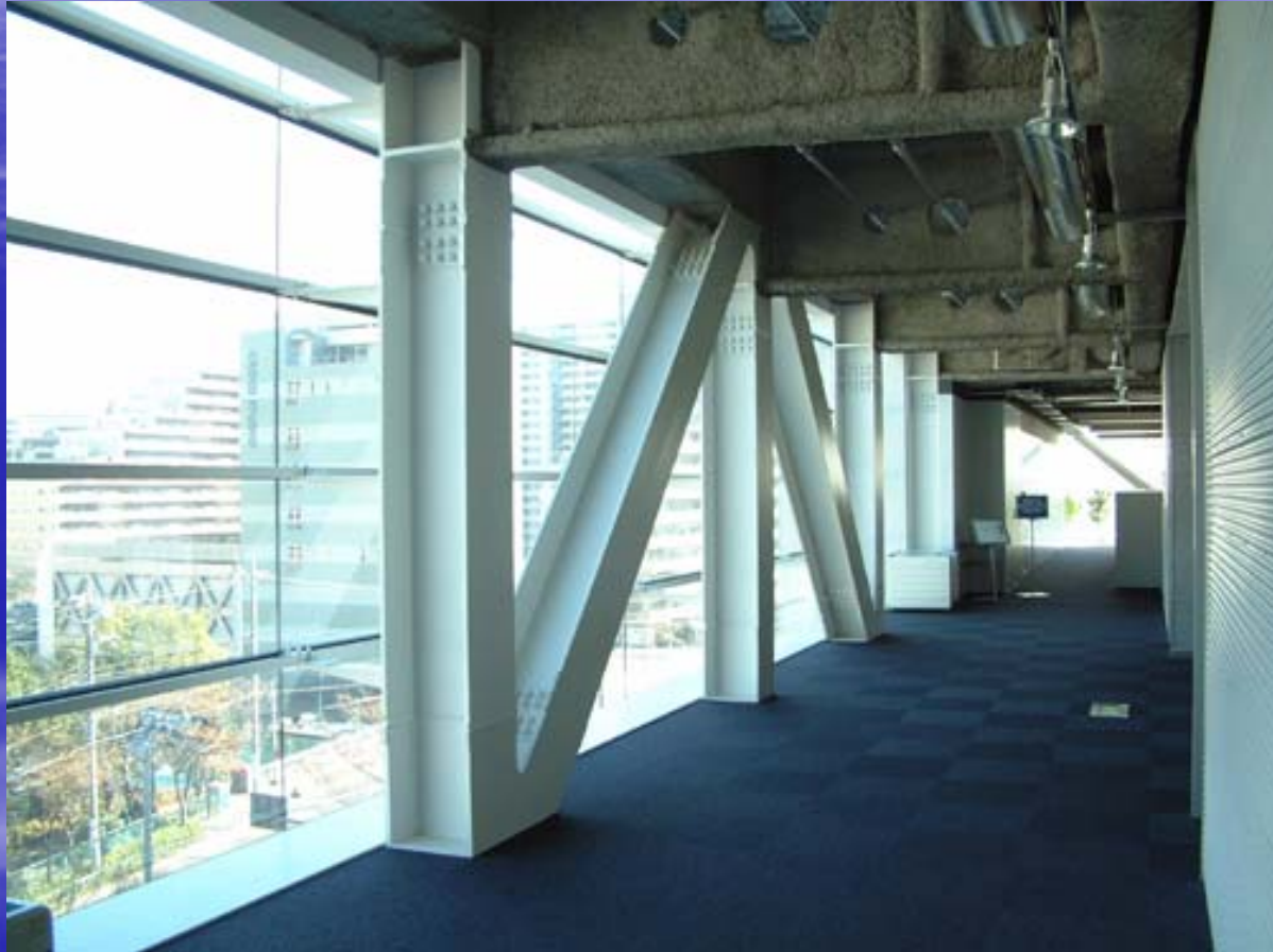
Frame without Fire Protection Covering Compartment of Elevator Hall using Water Curtain
